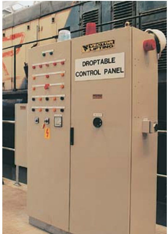
Typical Control Panel.
