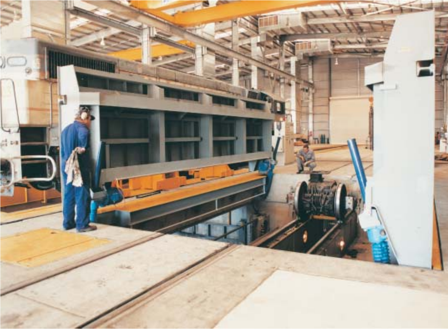
This photo shows the trafficable cover opened on the release track at Queensland Rail's Stuart Locomotive Maintenance Depot in Townsville, Queensland.
