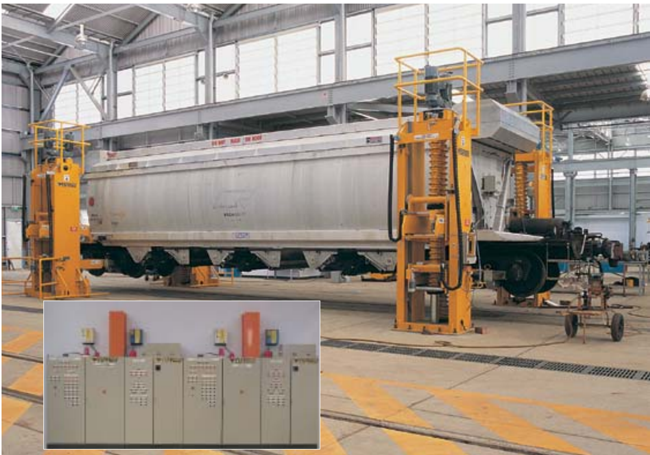
Another angle of the Willowburn facility, inset shows the ergonomic design of the control panel.
