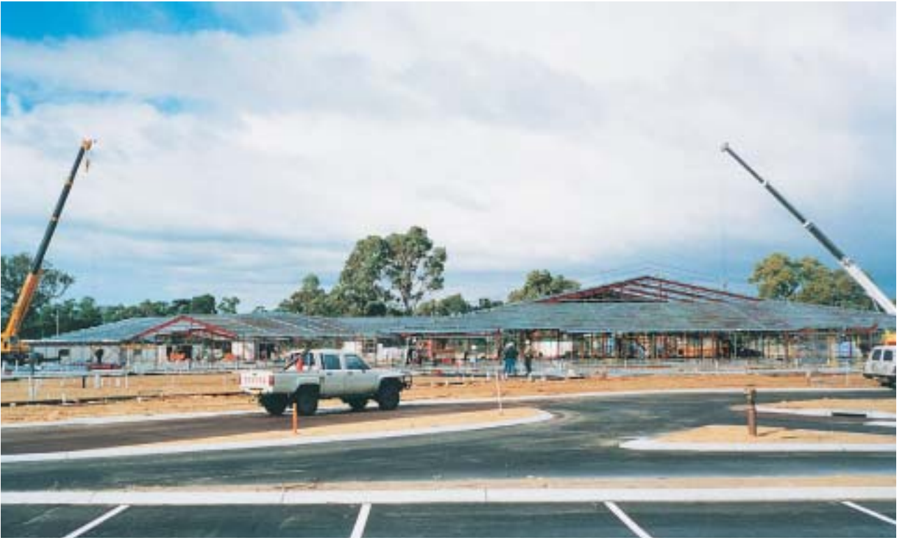
SCENNA CONSTRUCTIONS have a wide range of skills and expertise available to every client. This State Government hospital in the regional town of Mandurah in WA is an example of our civil construction work.
