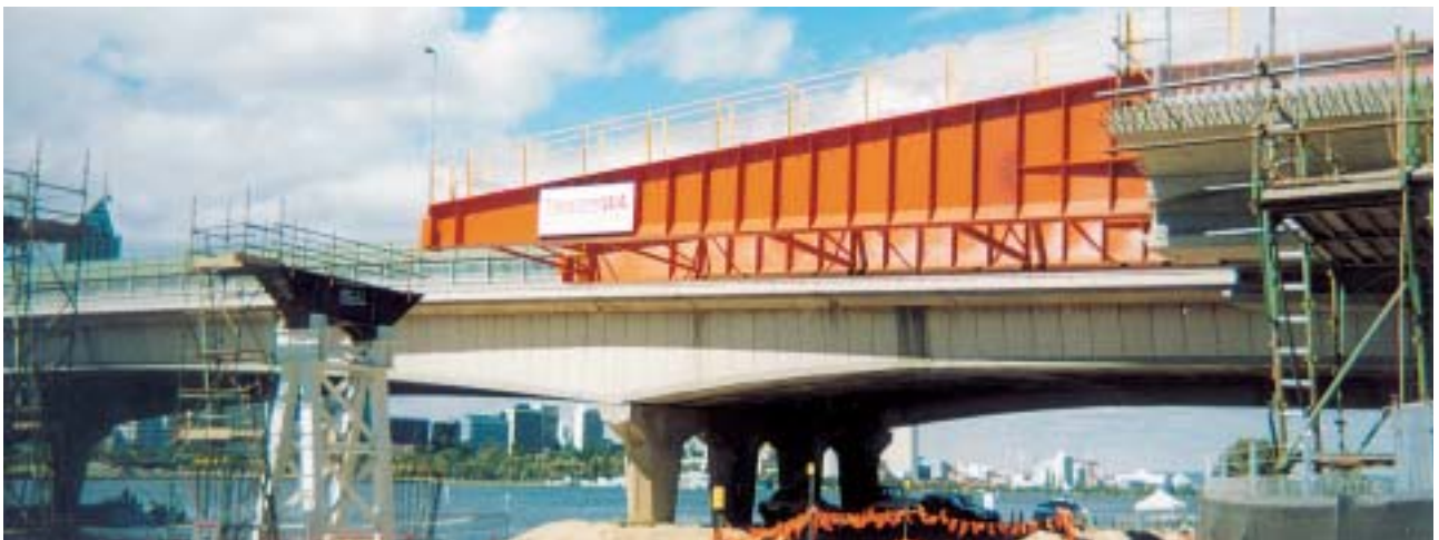
Perth's Narrows Bridge Duplication project featured an incremental launching system. Launching noses acted as guides and support during the incremental launching process over the Swan River. Temporary support piers are replaced with permanent piers once the spans are completely across the river.
